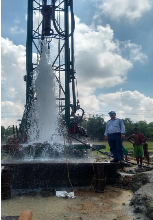
Fig 3.1 High Yielding well constructed by CGWB , ER, Kolkata in Alluvium formation at Sutia, Nadia district, West Bengal
