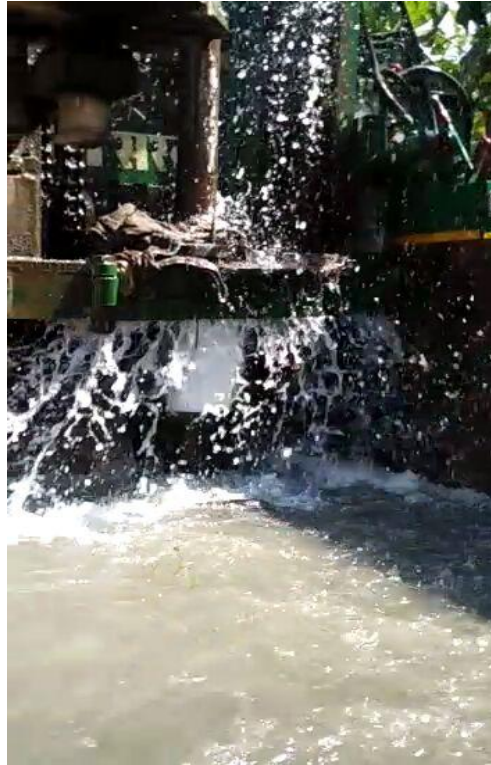
Fig 3.2 High Yielding well Kadambazhipuram Palakkad district, Kerala discharge 20lps
